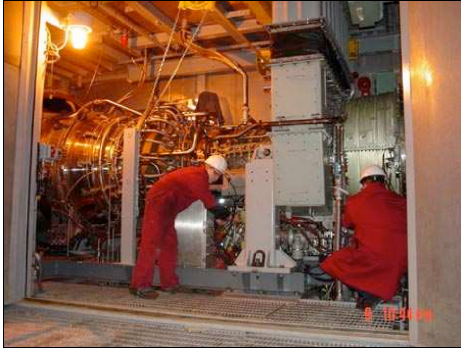
Figure 2-4: GE LM6000 Turbine Engine – Inside Turbine Enclosure 7
